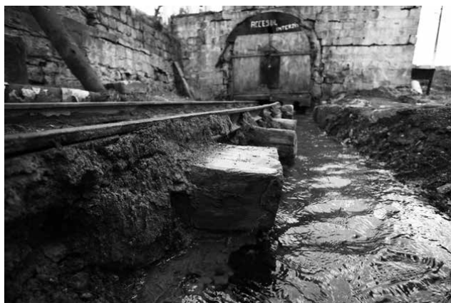
Fig. 1. Water drainage at 'Gura Minei' abandoned mining perimeter (23.05.2014, A. Lancranjan)
