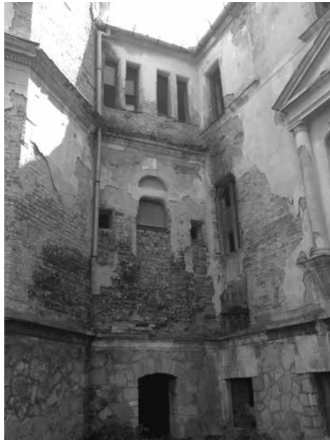
Fig. 1. Degradation of the installation of storm water discharge
