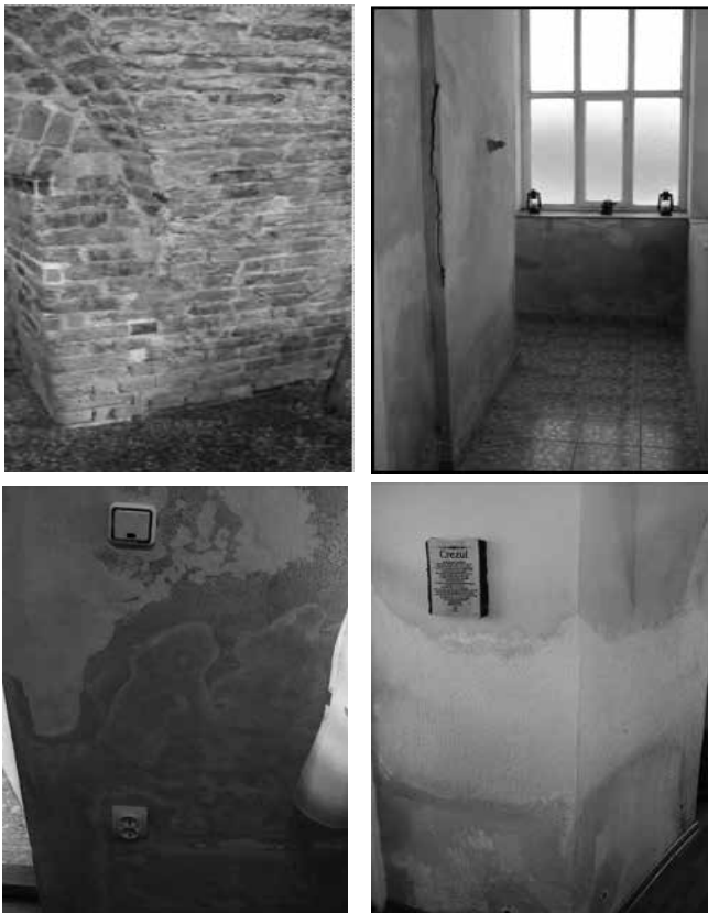
Fig. 1. Presence of the humidity: the basement, corridor, smoke room, living room
