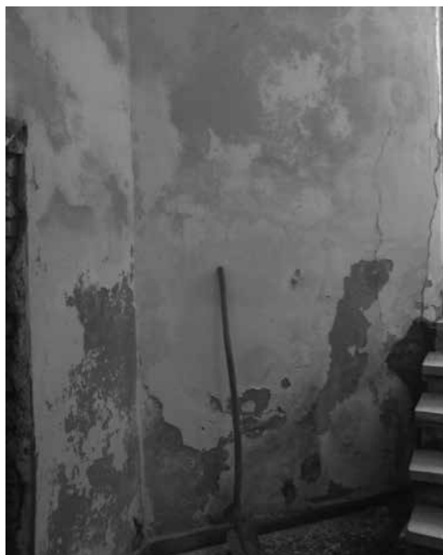
Fig. 2. Poor ventilation of the underground
