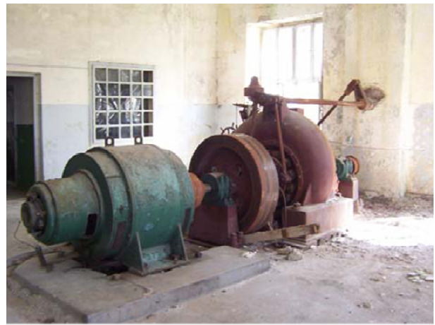
Fig. 10 Turbine out of function.
